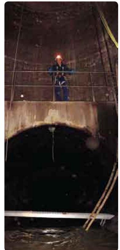
Maintenance of equipment in the sewer requires personnel to be trained in confined space entry.
