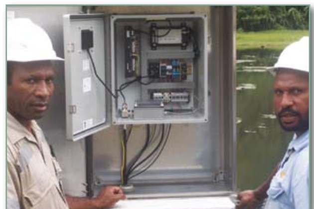
A double enclosure station design has improved equipment reliability.
